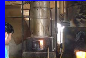
Boiler - Plywood unit, Ernakulum
